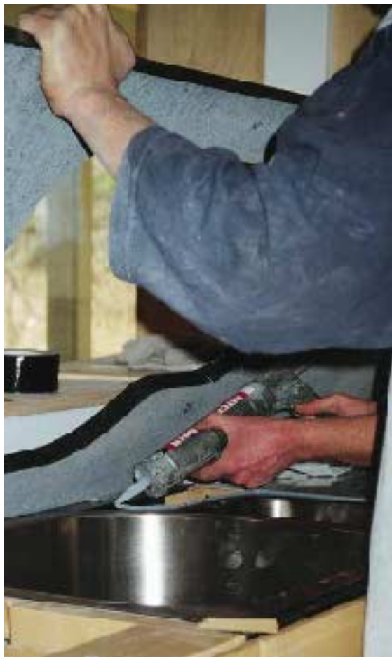
Figure 9. Before the stone countertop is lowered for the last time, a generous bead of silicone caulk is applied around the sink flange. This stainless steel sink is supported by custom-made angle-iron rails, which also help support the granite.
