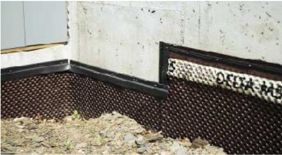
Figure 5. A plastic termination strip gets nailed along the flat tab at the top of the membrane (at right in photo). Where the flat tab gets cut off, as at this step-down, the cut edge is protected by a 2-inch-wide molding strip.
