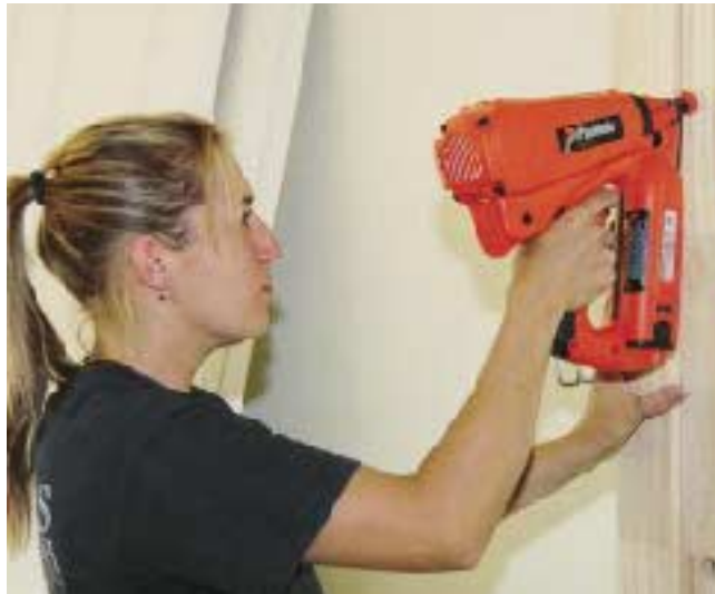
Figure 2. Carpenter Cori VanDyck uses the newest Paslode cordless finish nailer to install a door jamb. This nailer's light weight, compact size, and the absence of a hose are clear advantages for small jobs and pick up work.
