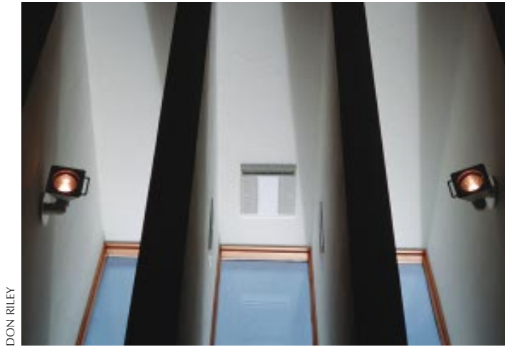
Figure 4. Three 20-inch-wide shafts defined by roof trusses are interconnected by heating louvers, allowing excess summer heat to be exhausted by a thermostatically controlled exhaust fan.
