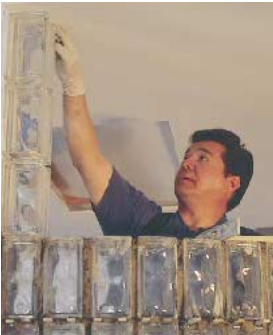
Figure 1. Because glass block cannot be cut, layout is crucial. Here, the author dry-stacks the last few courses to make sure he ends up where he planned.
