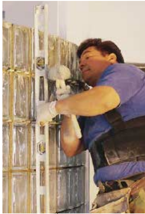
Figure 6. Every block gets trued with a torpedo level (left), while the 4-foot level measures the overall plumbness of the wall (right).
