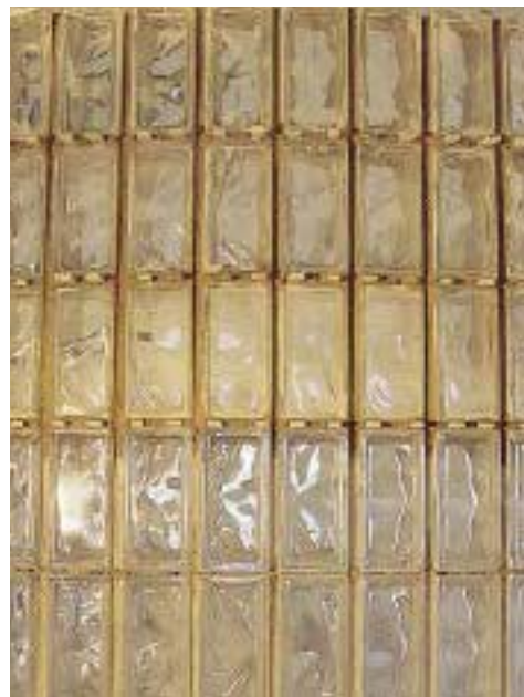
Figure 5. Three courses of block can be laid before waiting for the mortar to set.
