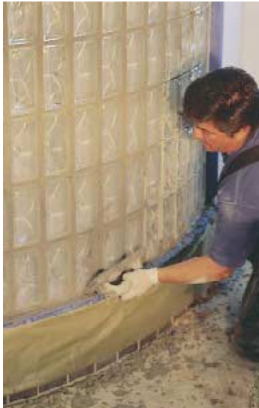
Figure 2. Masking adjoining surfaces at the beginning of a job saves a lot of cleanup time at the end.
