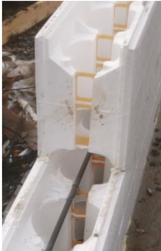
Figure 6. A preshaped wire wraps under the plastic web and over the rebar to keep the steel in place.
