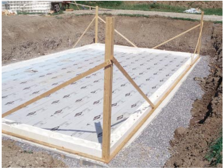
Figure 3. Plumbed and braced 2x6 corner bucks will hold the foundation dimensions as the walls are stacked. The 1x4 cleat attached to the footing keeps the first course from kicking out during the slab pour.
