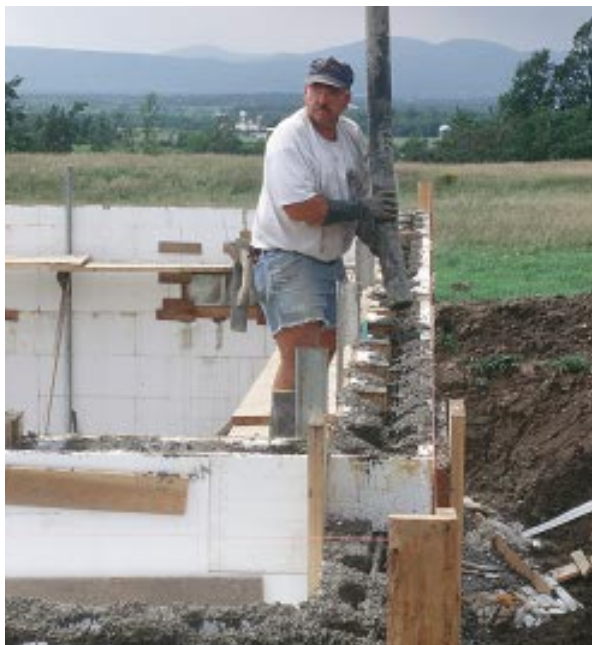
Figure 9. Moving the hose evenly around the forms ensures that the concrete is placed in shallow lifts. Note the steel wall braces against the rear wall, which support staging planks.
