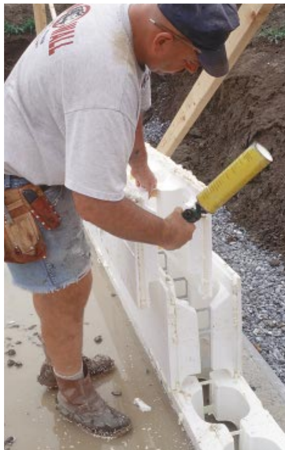
Figure 5. Aerosol urethane foam cements the tongue-and-groove connections between blocks. Note the plastic webs, which hold the sides of the blocks together and provide support for horizontal rebar.
