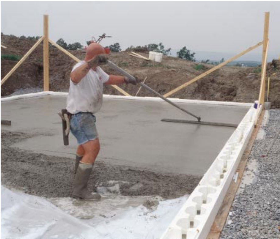
Figure 4. The first course of block acts as a form for the basement slab. The finished slab provided a level work surface, since the foundation is built from the inside.
