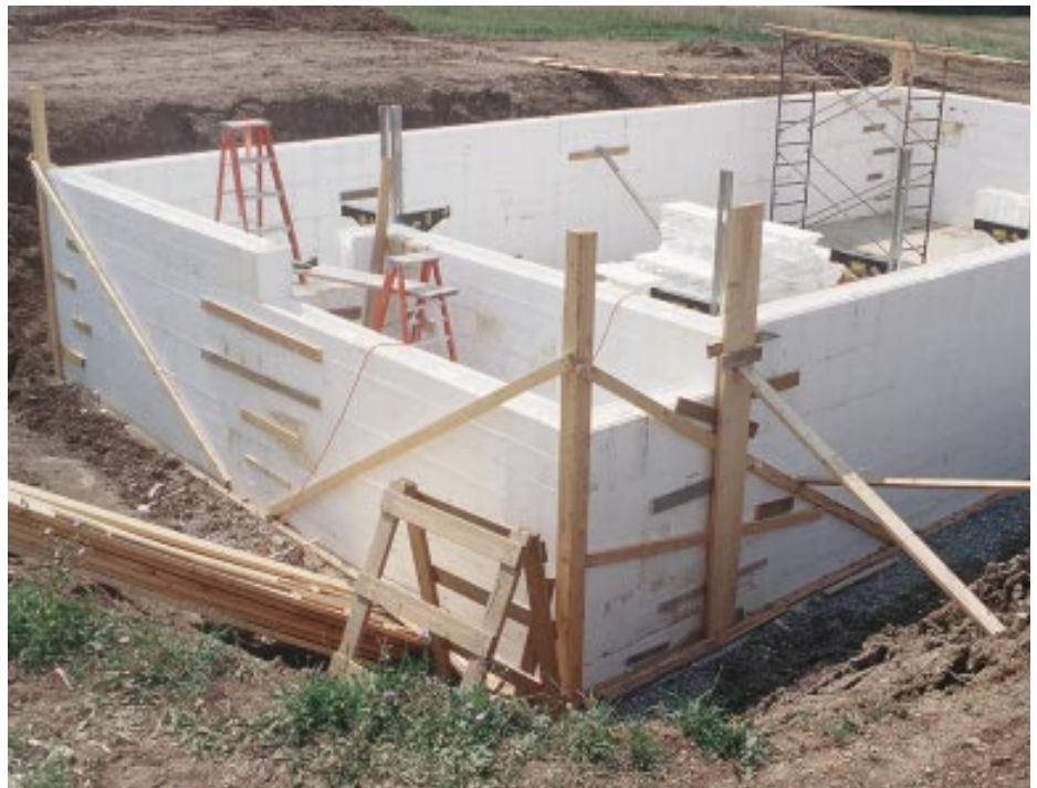
Figure 7. A vertical 2-by braced against the bank helps keep a wall intersection plumb. The wall braces, which can be seen behind the ICF wall, support staging brackets, which provide access for stacking the upper blocks and pumping the concrete.
