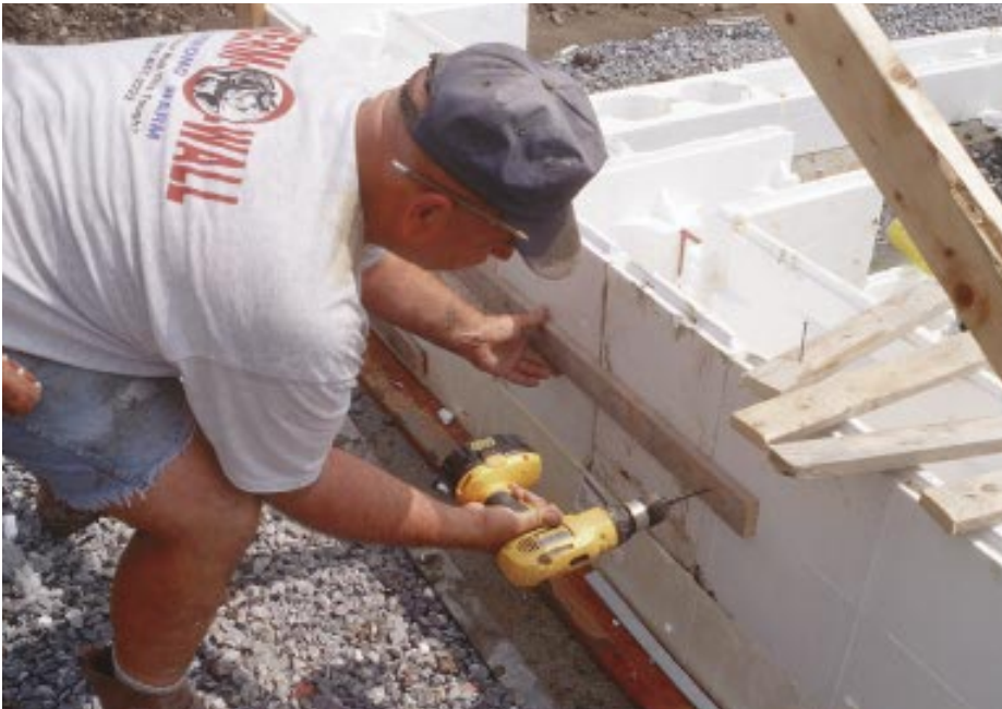
Figure 2. Lengths of 1x3 or 1x4 strapping are used to strengthen weak spots in the ICF forms. The strapping is screwed to the plastic tees embedded in the forms.
