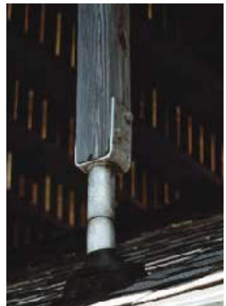
Making use of available flashing technology, the author designed this hold-down around a common plumbing vent roof boot.
