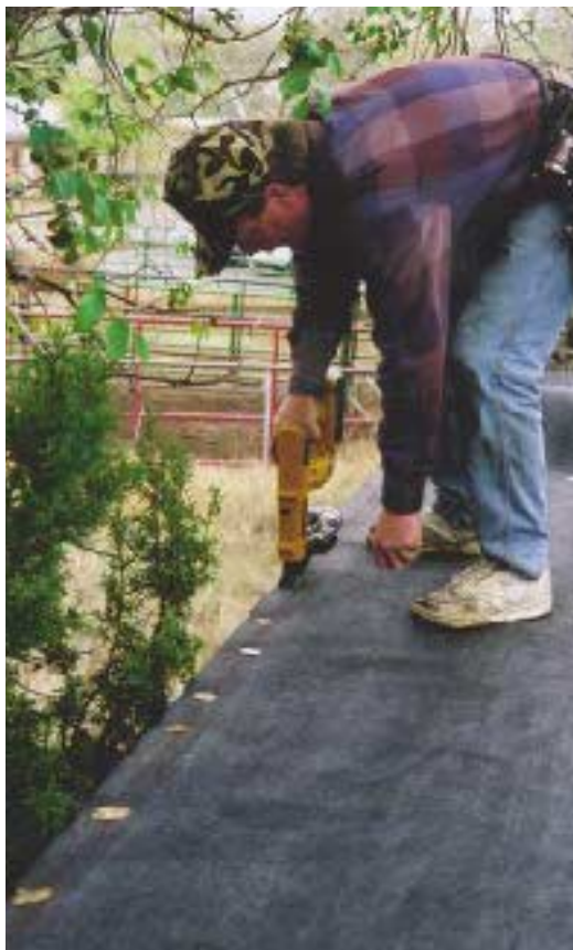
Figure 1. The base sheet is fastened to the deck with roofing nails and metal cap plates called shiners (right). Nails are spaced every 9 inches at edges and seams and on 12-inch centers in the field. Heated with the torch as it unrolls, the membrane fuses to the base sheet and to itself at seams (far right).
