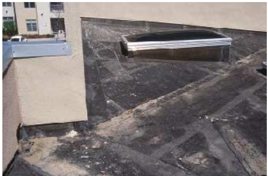
Figure 3. The large cricket in this parapet corner directs rainwater toward the roof drain. Note how the torchdown membrane runs up the side of the skylight well.
