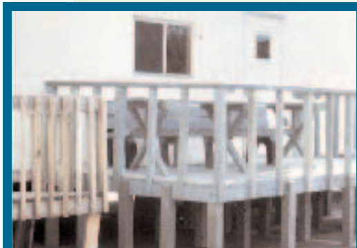
This 11-year-old plastic lumber deck at Rutgers University in New Jersey was recently tested by the ASTM, which found that the material used has gained strength and stiffness.
