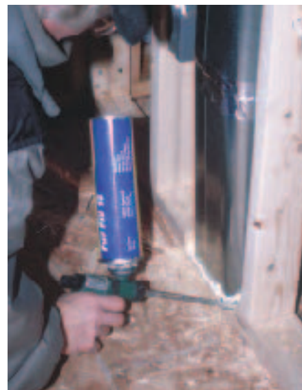
Figure 6. Where an oval duct penetrates a floor, aerosol foam helps secure the stack to the framing.
