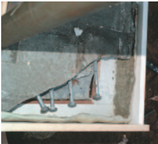
Figure 2. To repair a missing corner of the textured concrete floor, the crew first made a latex mold of the opposite corner. The mold was then used to line the small form, to capture the edge texture. Galvanized bolts were epoxyed in place to strengthen the new corner.
