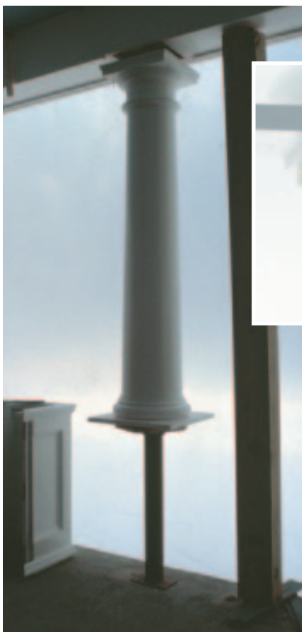
Figure 3. The first step in installing the columns was to slip the cedar column and the top of the pedestal over the screw jack post and position the jack (left). The cedar column was held in place with a clamp-on standpipe bracket, reinforced with a piece of marine plywood (above).
