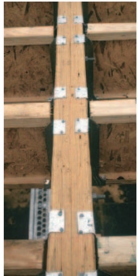
Figure 2. To avoid floor squeaks, the author maintains a 1/4-inch gap between the hung I-joist end and the engineered header and makes certain that all holes in the joist hanger are properly nailed.
