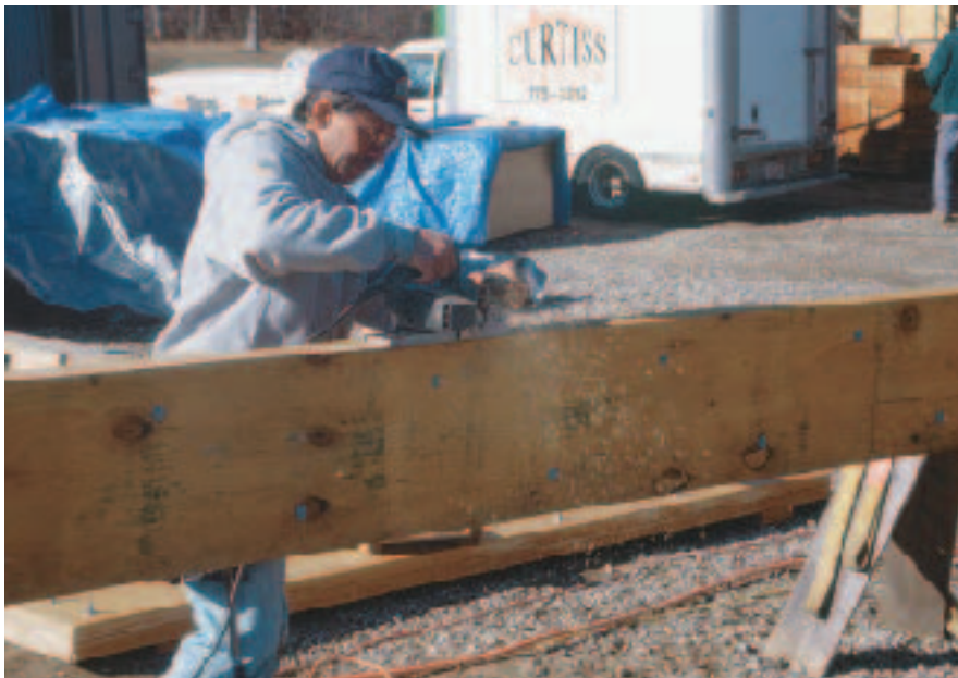
Figure 4. LVL planks are somewhat irregular in width. Power-planing the top edge of a built-up header eliminates some bumps in the road.
