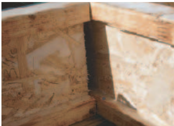
Figure 8. In some jurisdictions, the inspector may require a fireblock in the gap left where one I-joist butts perpendicular to another.
