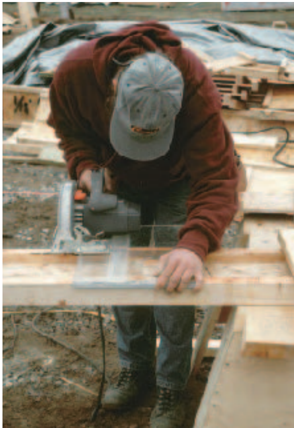
Figure 5. A thin plastic custom cutoff guide carries an 8-inch-diameter saw over the 2½-inch-wide flanges and recessed web without overly compromising the depth of cut.
