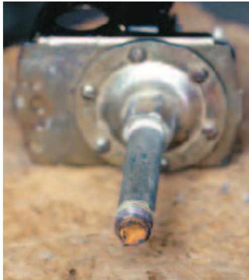
Figure 4. This galvanized pressure switch pipe is completely blocked with corrosion. As a result, the pressure could build to disastrous results or the pump refuse to turn on at all. A brass nipple would have prevented this corrosion.
