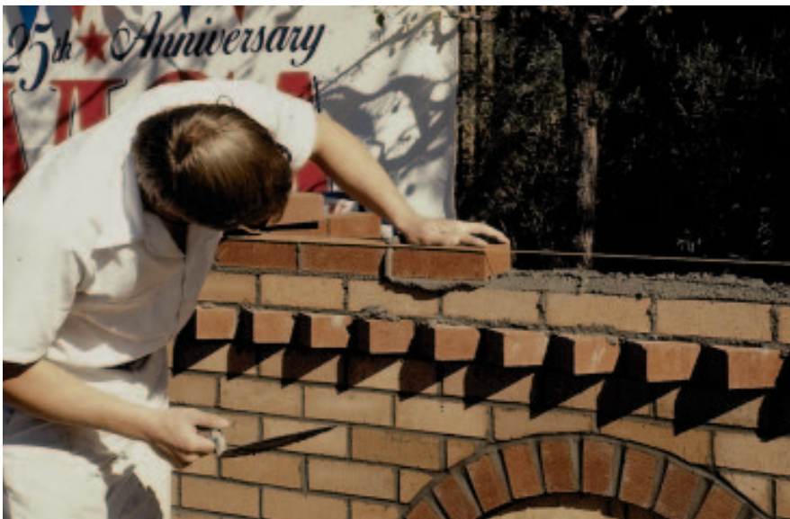
A mortar with good workability extrudes readily from the joint when the mason applies pressure to the unit.
