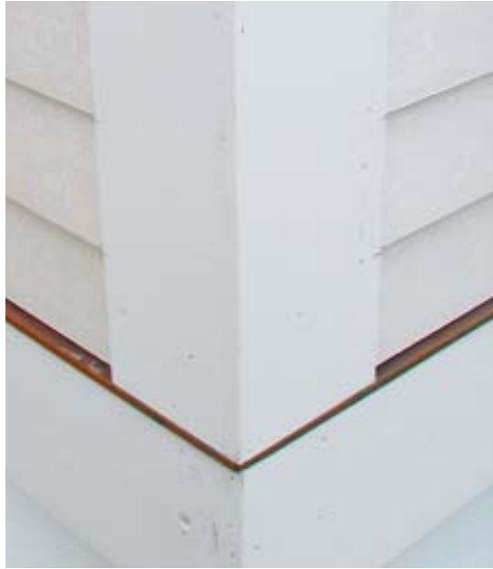
Figure 3. Gluing corner boards with PVC cement keeps joints tight and makes installation easier. The author's crew hides expansion gaps with a slight back-cut on the bottom of corner boards where ordinary gaps would be more obvious.
