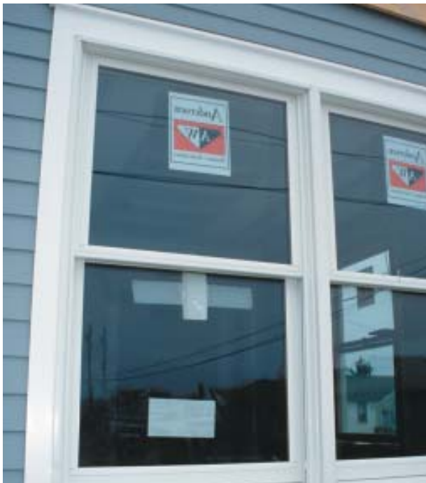
Figure 9. After the pre-assembled casing is nailed in place over the window fin, the narrow expansion gap between trim and window is caulked. Although the manufacturer claims that the material can be left unpainted, two coats of acrylic latex leave subtle brush marks, for a thoroughly convincing "wood-like" appearance.
