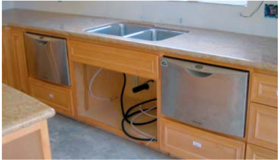
Figure 1. A pair of single-drawer Fisher & Paykel dishwasher units solve the problem of fitting a standard unit beneath a countertop of substandard height.
