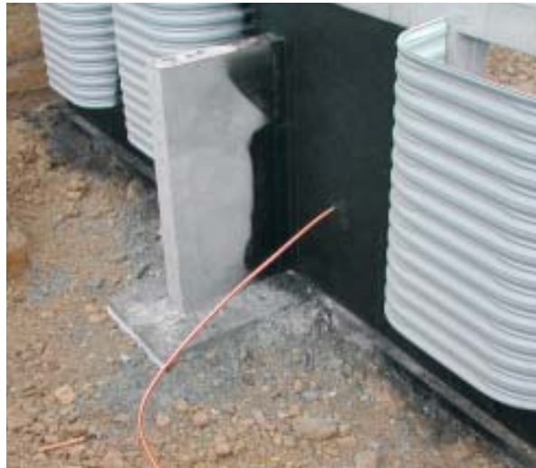
Figure 5. Large basement windows provide light and air and satisfy egress requirements but reduce the foundation’s ability to resist lateral soil pressure. Reinforcing buttresses, or counterforts, are used where needed to provide added strength.
