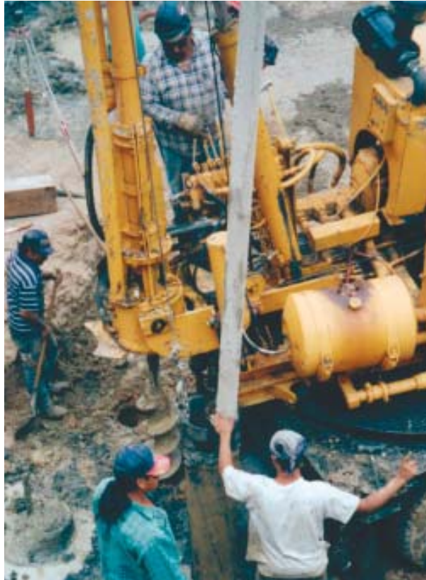
Figure 3. Where caisson boreholes extend below the water table, a temporary steel casing is inserted as the holes are bored. The casing is withdrawn as concrete is pumped into the borings.
