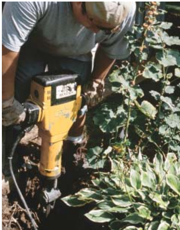
Figure 3. When the original posts are set in concrete, removing them takes time and may leave an oversized hole that requires extra concrete to fill. Breaking up the old base with a rented electric jackhammer saves time and trouble.
