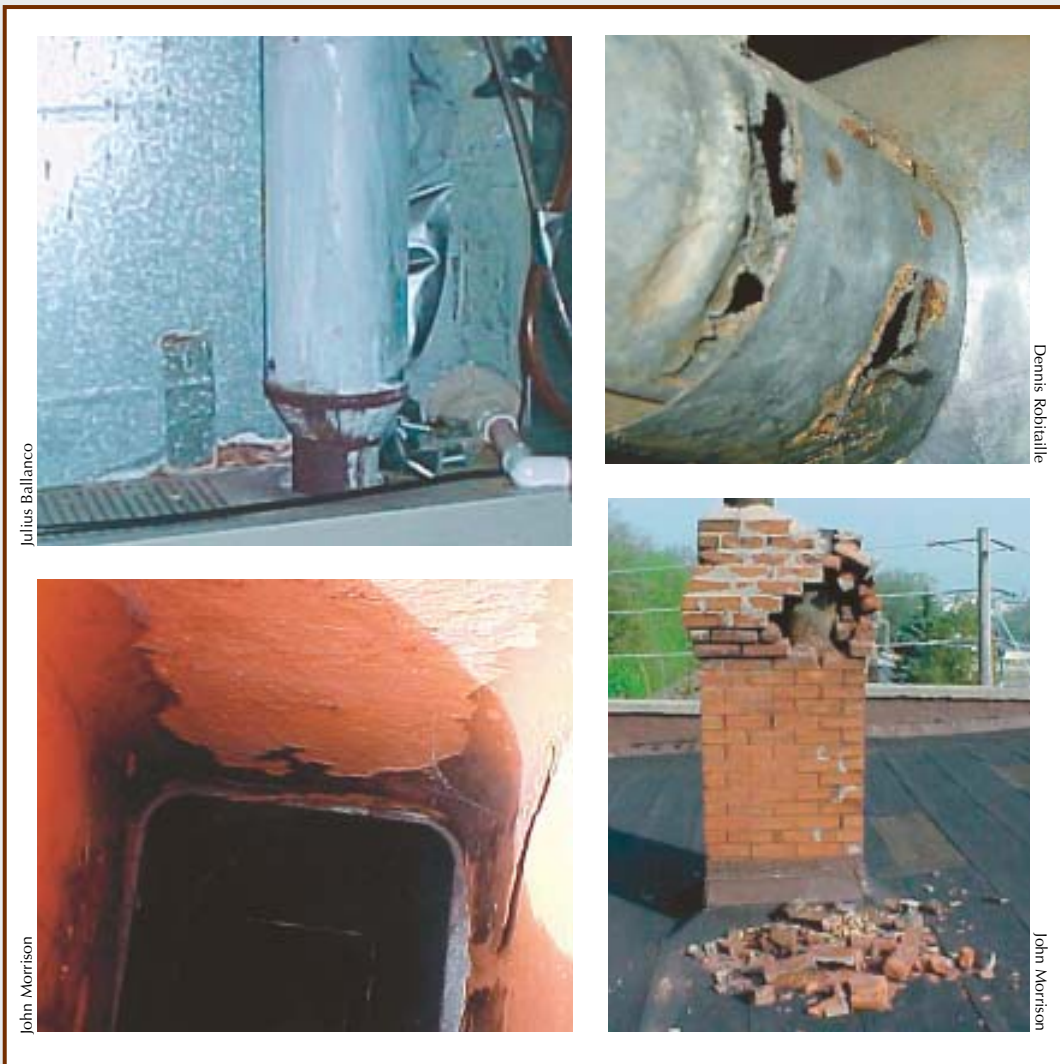
Figure 1. Condensation in gas flues is acidic and can attack vents and chimneys. Telltale white deposits and rust are signs of corrosion (top left), which can perforate vent pipe and allow fumes to leak (top right). Chimneys are especially vulnerable: Acidic condensate eats through tile flue liners (bottom left) and destroys brick masonry (bottom right). It takes 50,000 Btus to heat a masonry chimney above the dew point of gas appliance exhaust, while only 125 Btus are needed to warm a B vent flue.
