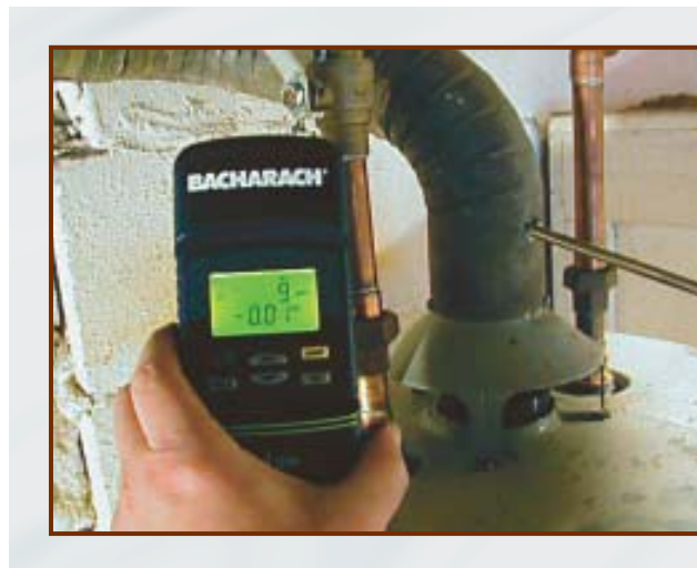
Figure 8. Modern test equipment can measure flue gases and analyze appliance performance in real time. The instruments will detect poor draft in the flue or combustion problems and help technicians pinpoint the cause.
