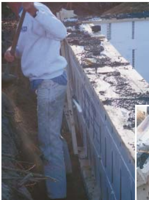
Figure 7. Inadequate bracing at a spliced form and a too rapid pour in one area caused a section of form to bulge outward (left). The affected area was located partway up a low section of wall, so the damage was contained by tamping backfill against the bulging form (below).
