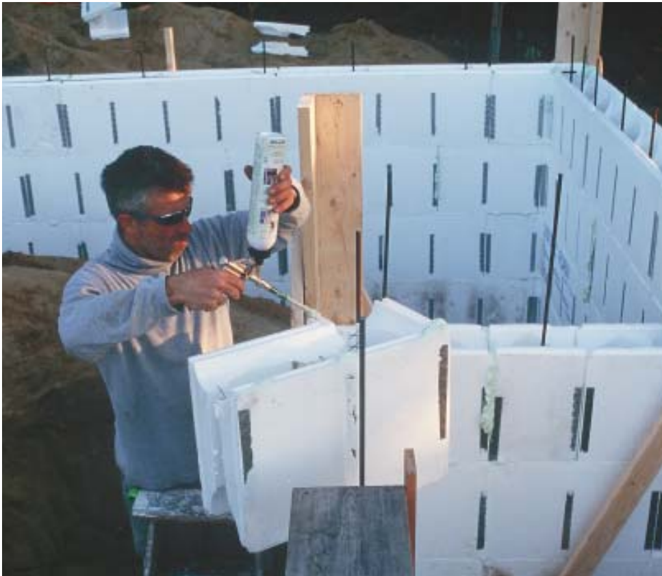
Figure 2. Walls are stacked one course at a time; corners are laid up using alternating left-hand and right-hand corner blocks. Polyurethane foam is used as “glue” between trimmed forms that lack the usual tongue-and-groove connection, but added exterior reinforcement is also needed in those areas.
