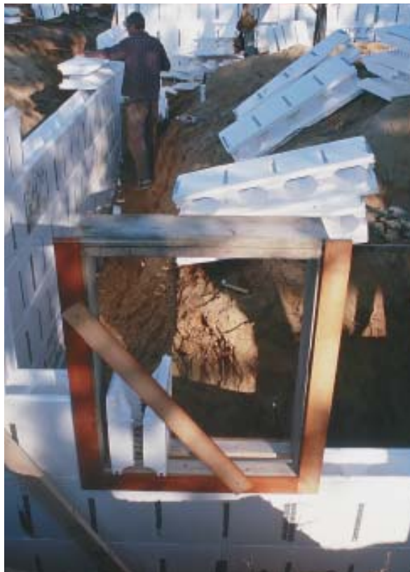
Figure 4. Window openings are created with simple site-built window bucks made from pressure-treated 2x10 stock. A slot between the two spaced 2x4s that serve as the bottom sill makes it possible to pour concrete into the forms below the window opening. Temporary wooden flanges help position the bucks (the inside flanges are not yet in place in this photo), while added exterior bracing keeps them plumb during the pour.
