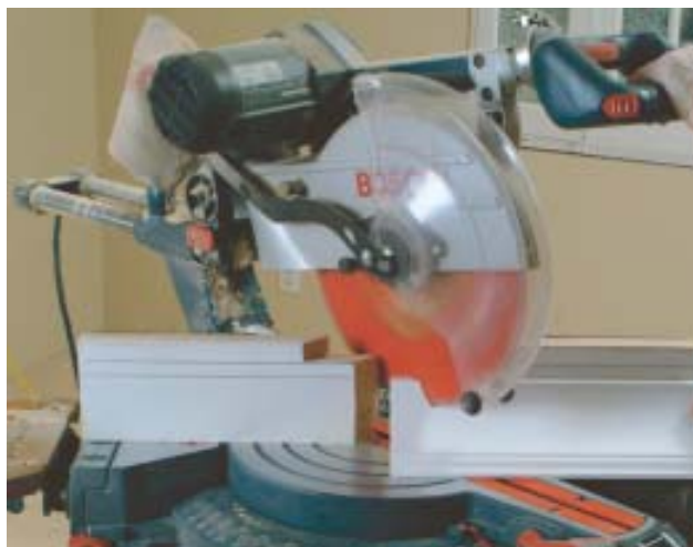
Figure 5. When cutting the transition piece, the first cut, made on the edge that meets with the level run of crown molding, is made in upside-down position — a standard inside corner cut (left). The other edge, which mates with the rake crown, is cut right side up (below).
