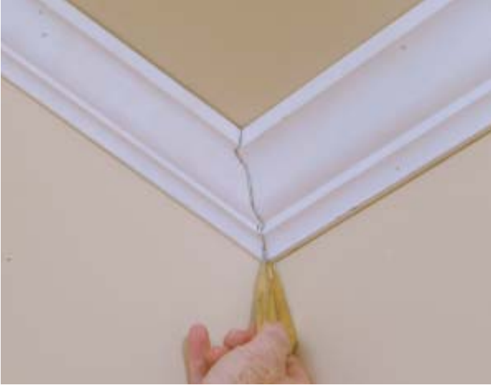
Figure 3. Using two sizes of the same profile — wider stock for the horizontal run, narrower for the rake — can sometimes work to turn a cathedral corner. The horizontal run still has the same spring angle, so the bottom doesn't have to be rebeveled, only the top, to match the slope of the ceiling.
