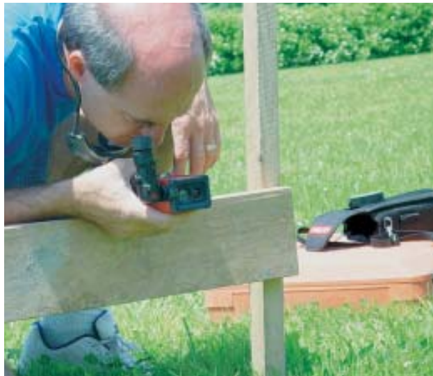
Figure 3. Laser measuring devices are great for layout and squaring because you don't need two sets of hands, and neither wind nor a sagging tape will affect the measurements. The author found that having a good scope helped with these tasks because it made aiming the device at a pencil mark much easier.
