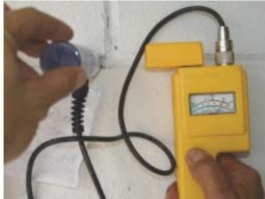
Investigators from Tampa, Fla.-based Construction Moisture Consulting sprayed water on the exterior walls of 10 Florida homes. Within minutes, interior moisture readings maxed out at garage-wall mortar joints (left) and living-space drywall. Soon, water was visibly trickling down block wall faces (below left) and seeping out from behind baseboards (below).
