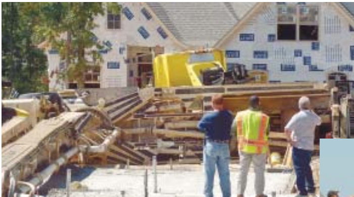
This concrete pump truck tipped over on a job site in Lake Caroline, Miss., pinning a worker beneath the boom. OSHA is investigating.
