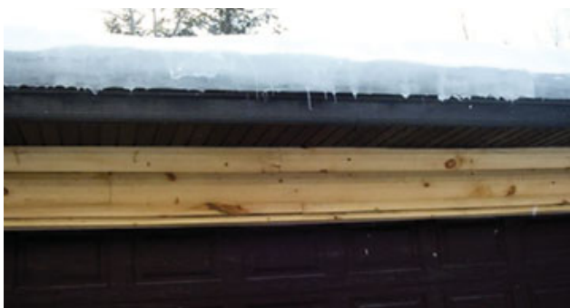
Figure 1. Ice dams on this new home in Michigan's Upper Peninsula formed above interior cathedral ceilings, which were insulated with low-density open-cell spray foam and were unvented. The roof sections with no ice are above unheated areas of the home.
