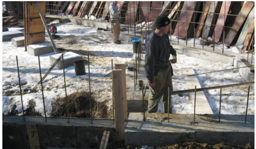
Figure 3. For the 10-inch-thick foundation walls, the engineer specified a grid of #5 rebar. The footings step down 5 feet on the walk-in side of the foundation. Because this portion of the wall is not subject to soil pressure, its thickness is reduced to 8 inches.
