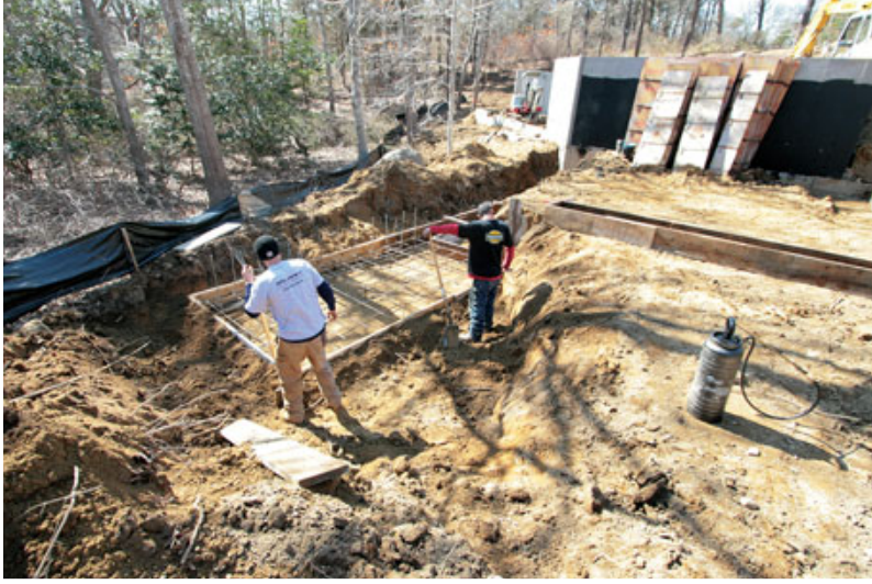
Figure 6. One crew began installing the septic system while another formed the attached garage foundation. The heavily reinforced spread footing (left) will anchor a retaining wall that extends from the back wall of the garage (below).
