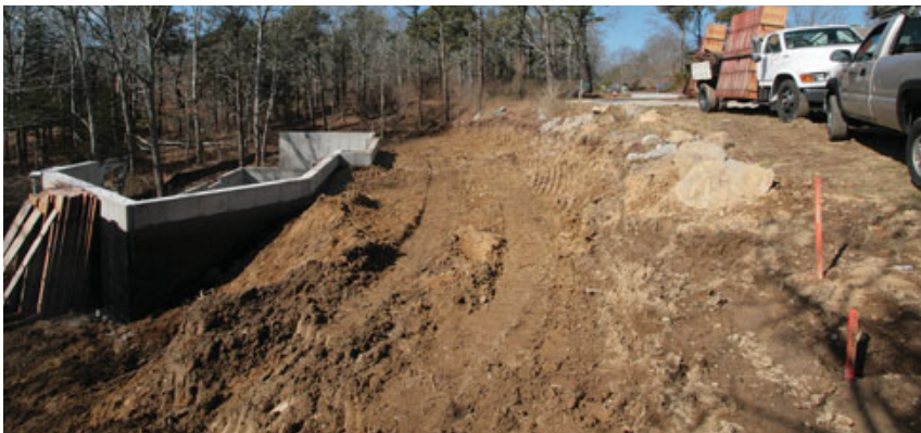
Figure 5. The authors installed drain tile, which outlets to daylight around the completed foundation (top). Note the standing water just inside the silt fence. A section of the lot between the foundation and the street above was then backfilled to provide the required level base for the septic system (above).
