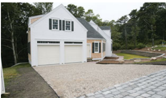
Figure 7. A dry-laid masonry retaining wall and hard-surfaced walkways, installed as soon as possible after the completion of foundation work, provided early curb appeal and a mud-free site throughout the rest of the project.
