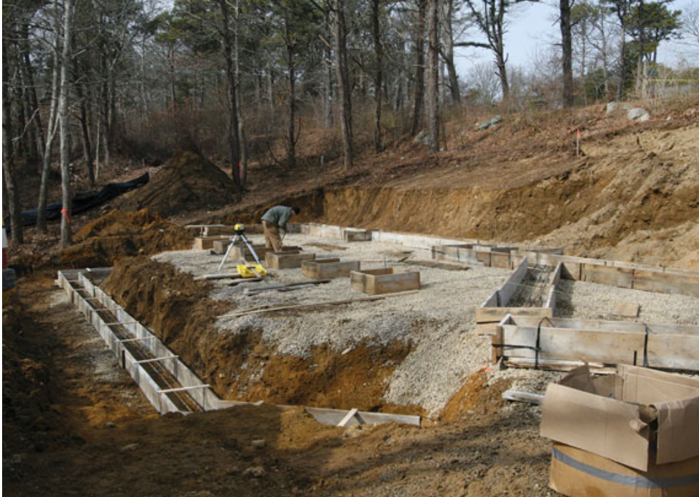
Figure 2. To improve traction for workers, the authors spread stone over the wet clay soil. Footing forms were placed on top of the stone.
