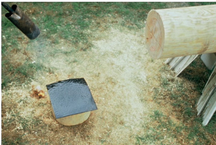
Figure 5. A propane torch heats torch-down roof membrane, used to prevent water from wicking up the log and causing rot. Once heated, the membrane is adhered to the bottom of the log post and trimmed to fit exactly.
