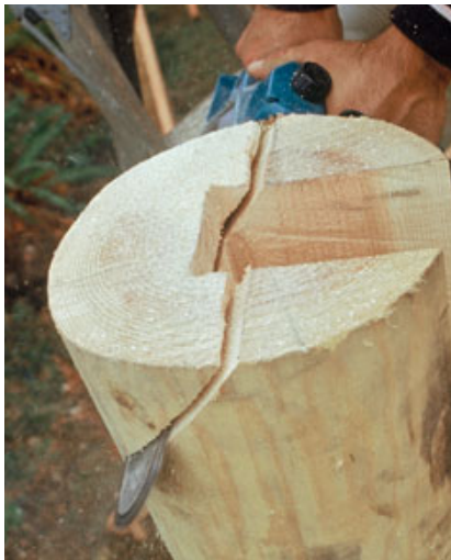
Figure 8. After the pockets for the beams are cut, the tops of the posts are beveled so that they shed water.
