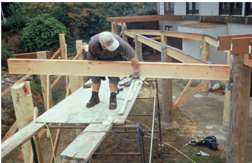
Figure 9. The author treats the wood with a borate preservative before placing the beams in their pockets. Note the torch-down roofing membrane applied to the beam and post tops in the background.
