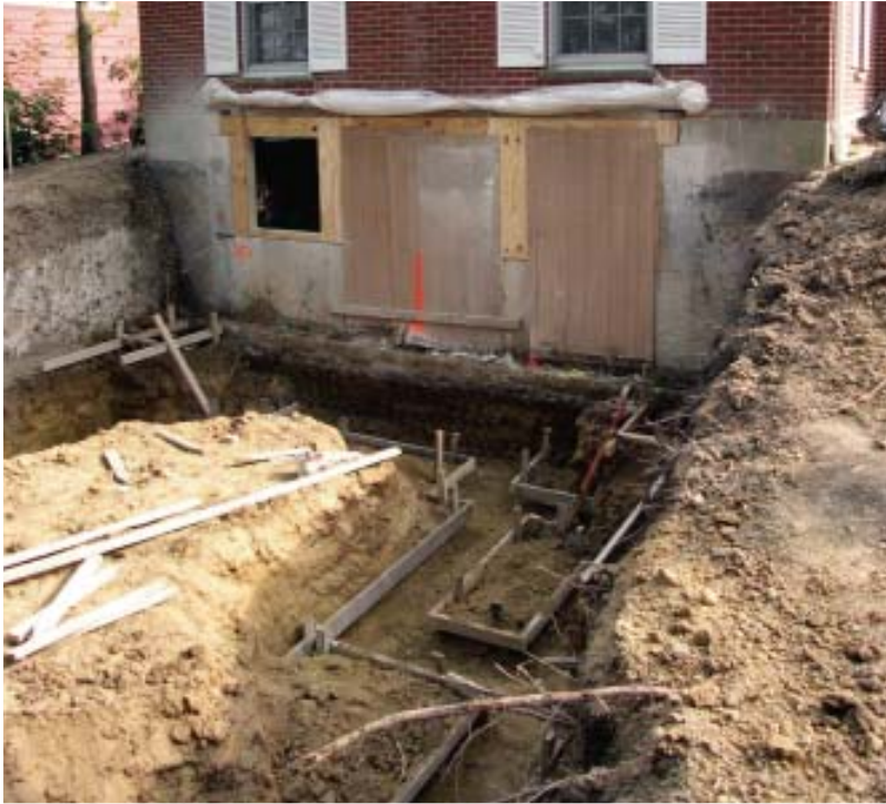
Figure 6. The footing below the patio door was dropped almost 4 feet to reach below the frost line; a one-sided form was used to pour that section of the foundation. Access was limited, so the crew used a bucket on a skid-steer loader to place the concrete for the footings; the walls were pumped.
