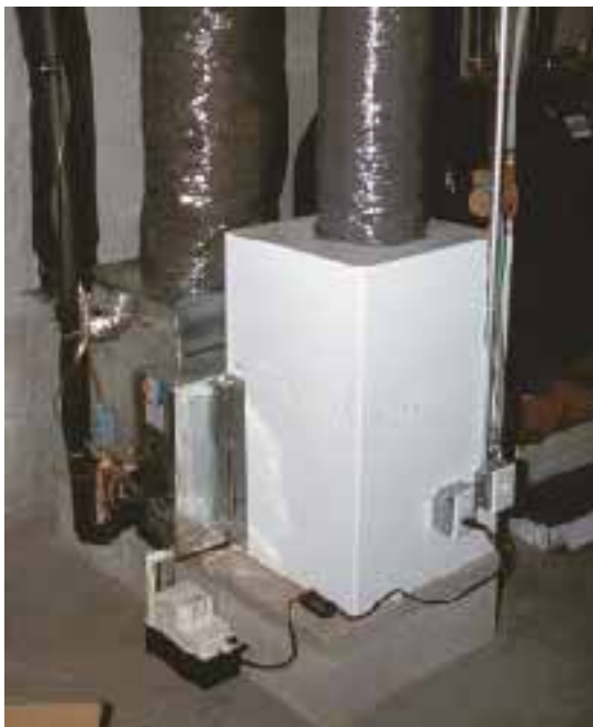
Figure 3. The system's air handler, or blower unit, can be installed in a horizontal, hi-boy, or counter-flow attitude and located to maximize usable floor space. A conventional system isn't as lenient in its placement.
