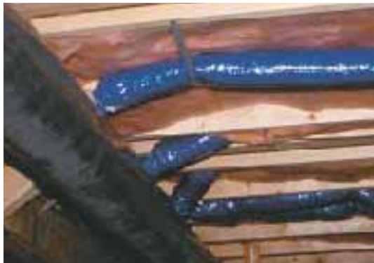
Figure 6. A single-diameter, minimally sized plenum stores and distributes pressurized air to the branch ducts at an equal rate. A conventional system relies on progressive step-downs in the size of the main trunk to maintain a relatively equal volume of airflow at each vent, making installation far more labor intensive.
