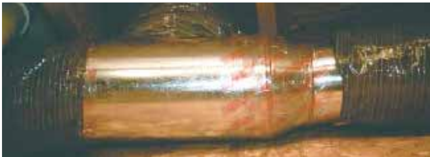
Figure 7. Airtight ductwork is absolutely essential to the function of a high-velocity system. The author seals every joint in the ductwork with a clear, SMACNA-rated tape. Careful and attentive application ensures an airtight joint and makes leak testing unnecessary.
