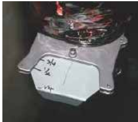
Figure 9. The author uses a standard blast gate to regulate fresh, outdoor makeup air entering the return plenum at a rate of about 10% of the total volume. Return air is drawn through a HEPA filter and conditioned before being returned to the living space.
