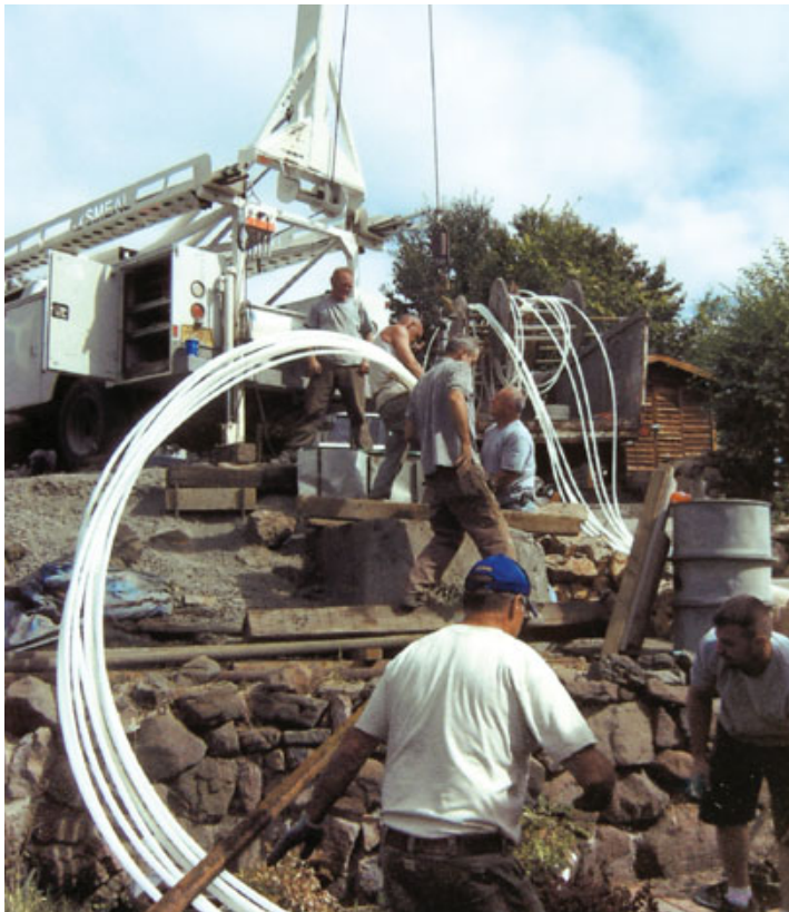
A well-drilling crew lowers a bundle of PEX piping into a thermal well that will heat a Klamath Falls medical office. Black iron pipe, long the traditional choice for downhole heat exchangers, tends to corrode in the hot mineral-rich groundwater, and typically must be replaced every 20 years or so.
