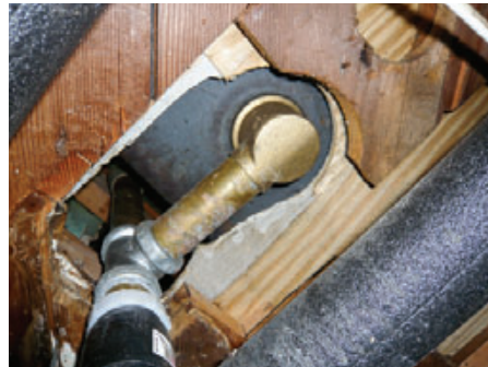
Figure 4. Floor openings around bathtub P-traps can leak as much air as an open window (above). They're best closed off with a piece of polystyrene — notched on one edge to fit around the pipe — set in a fresh bead of canned foam. A small filler piece at the drainpipe is foamed in place to complete the seal (right).
