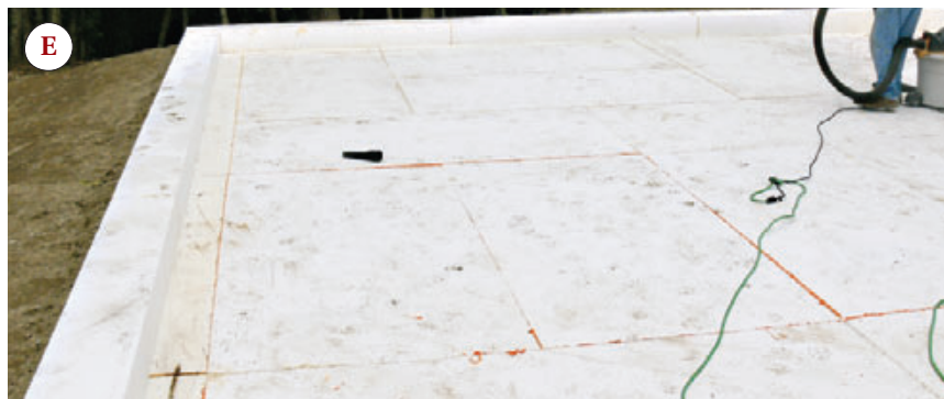
Figure 1. Custom-manufactured polystyrene served as the form system for the home’s 8-inch reinforced “raft slab.” The pieces were factory-cut with interlocking profiles (A) and a taper that serves as a draining wing insulation (B). The crew assembled the insulated forms on site using PUR Stick adhesive (C, D). A carefully compacted bed of crushed stone provided a flat sub-base for the insulation directly under the slab (E).
