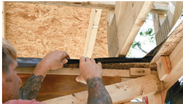
Figure 7. At the top plate of the upper-story wall, an OSB gusset projects inside to provide a taping surface for air-sealing the eventual interior ceiling.
