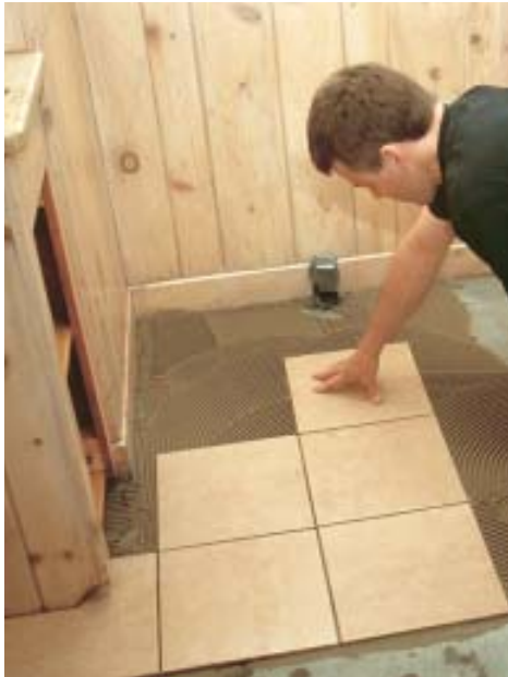
Figure 6. After curing for 48 hours, the mud base is ready for a standard tile installation. The author uses latex-modified thinset to adhere the tile.
