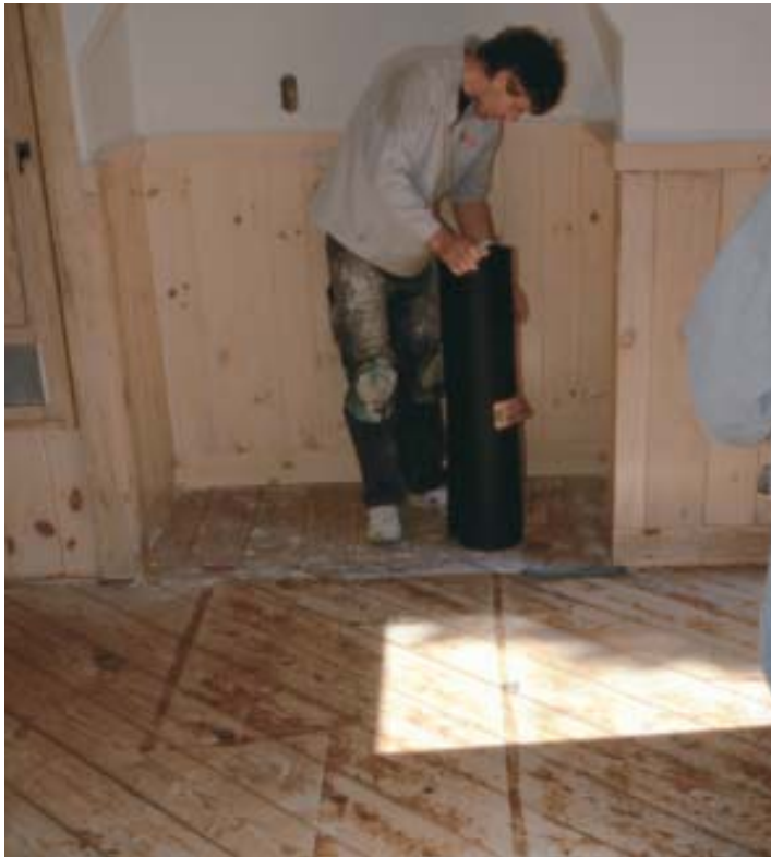
Figure 1. Although structurally suitable for tiling, this diagonally laid plank subfloor presented irregularities in plane that would telegraph through plywood underlayment and interfere with tile placement. A mortar base, or mud job, evens out the high and low spots, making an ideal tile bed.
