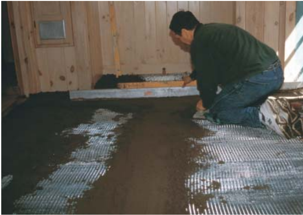
Figure 4. The primary “boss line” of screed establishes the mud bed level between critical points — in this case opposing door openings (left). Subordinate lines are then extended and leveled to establish the overall floor plane (below).
