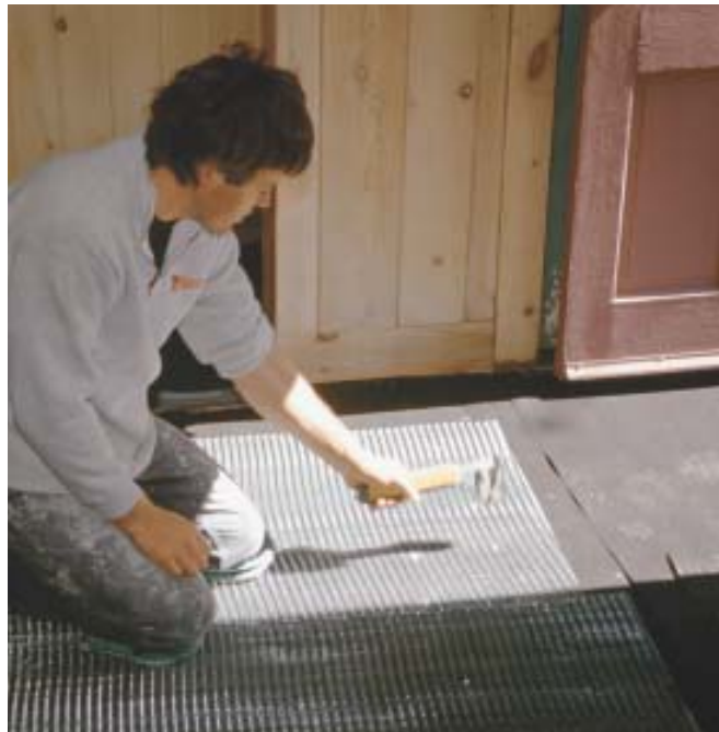
Figure 2. After covering the floor with 15-pound asphalt felt to retain curing moisture in the mud bed, the author staples reinforcing galvanized wire mesh over the entire surface.
