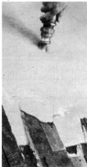
Gypsum-based underlayments, such as Gyp-Crete, shown here on a rehab project, are flexible enough that they can go directly over wood without metal lath. In new multifamily construction, gypsum toppings are used to improve fire and sound resistance of wood floors. Gypsum toppings can range from 3/4- to 3-inches thick.
