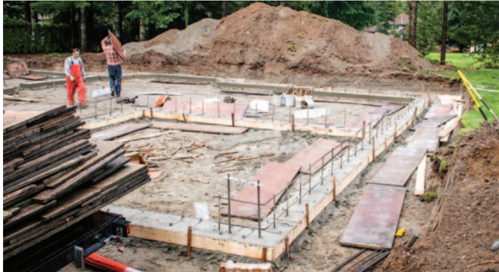
Figure 1. Workers finished up the steelwork before scattering the heavy Ply-form panels, with one continuous row of horizontal rebar about 3 inches up and another row at the top of the verticals.
