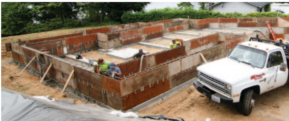
Figure 3. To build 4-foot or 6-foot-tall foundation walls, the author stacks his forms horizontally on snap ties laid across each lower course. Aligning the stacked panel joints vertically speeds installation and makes it easier to strip the forms later.
