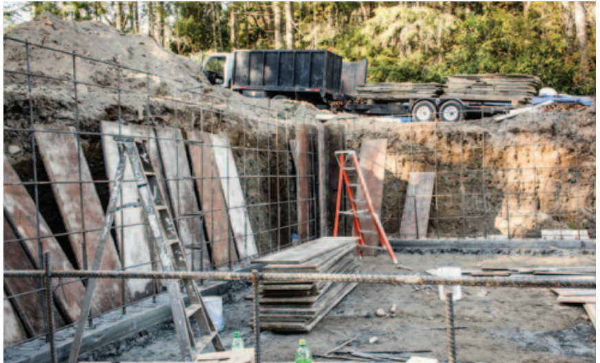
Figure 2. Reinforcement schedules for tall walls typically call for horizontal rebar on 12-inch to 18-inch centers depending on site conditions and structural requirements.
