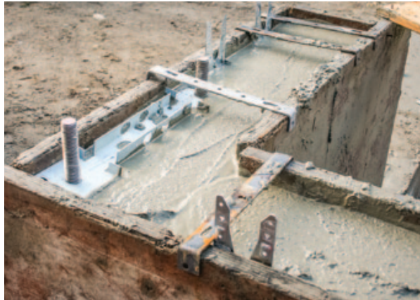
Figure 7. The author prefers Simpson MASA mudsill anchors over traditional anchor bolts for fastening the framing to the foundation. In the rush of the pour, this shear brace template was installed upside-down, so the author will just pop it out after the concrete has set up.
