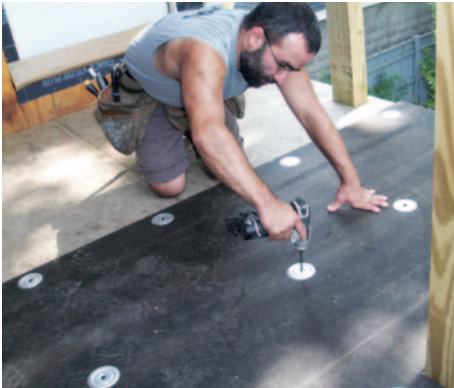
Figure 2. To protect against fastener show-through, the author added a layer of wood-fiber recover board, fastened to the structural deck with the same reinforced galvanized screw plates and 1 5 / 8 -inch screws used to secure the TPO membrane.
