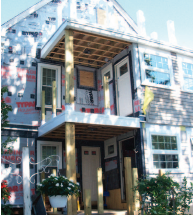
Figure 1. Using a membrane on all three decks ensures that water from rain or snowmelt will drain away from the house. On the ground-floor deck, the membrane keeps water away from the foundation, protects the underlying framing and connections, and allows for dry storage underneath.
