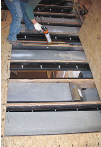
Figure 3. The engineer's plan called for steel reinforcement — plate steel and C-channel — to be bolted to the existing floor joists (above and left). The old subflooring was replaced with \frac{3}{4} -inch AdvanTech T&G sheathing glued and screwed to the framing (below).
