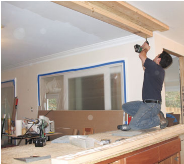
Figure 6. To anchor the hanging peninsula cabinet, a crewmember fastens double 2x6 cleats to the ceiling framing with structural screws and glue.
