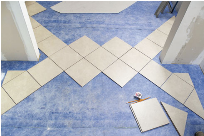
Figure 10. Once the membrane has been installed with Noble's contact-type adhesive, tile layout and installation should follow as soon as possible to lessen the risk that the membrane surface will get dirty or damaged.
