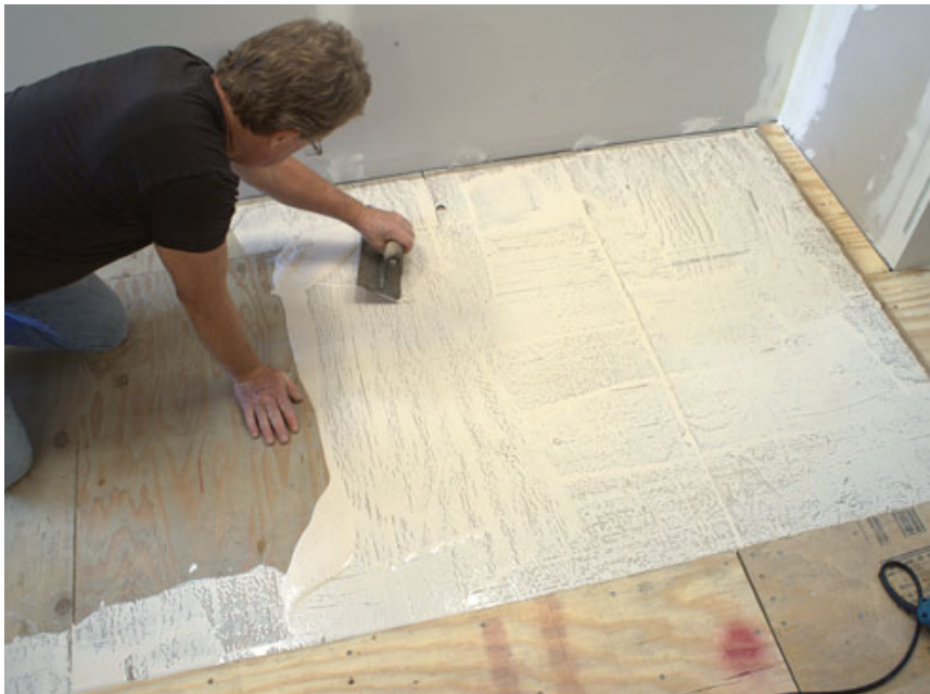
Figure 3. To achieve maximum strength and smoothness, 95 percent to 100 percent of the entire plywood surface must be covered with ANSI Type 1 or 2 water-resistant wood glue. At the perimeter of the floor, to avoid squeeze-over into the movement-joint slot, the author keeps the glue about 1/2 inch from the wall.
