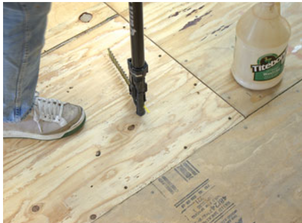
Figure 5. Using a stand-up screw gun with quick-loading 22-screw clips is substantially faster than shooting individual screws. It's also much easier on the knees.
