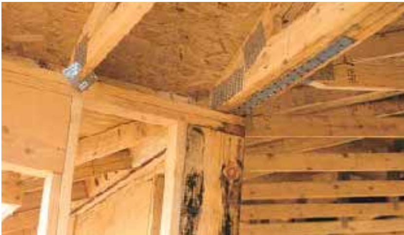
Figure 2. The strap in the photo above carries tension forces from the collector truss to the shear wall beyond (lower left in the photo). In the photo at top, straps running in both directions connect the wood I-joist second-floor framing to the shear walls below.
