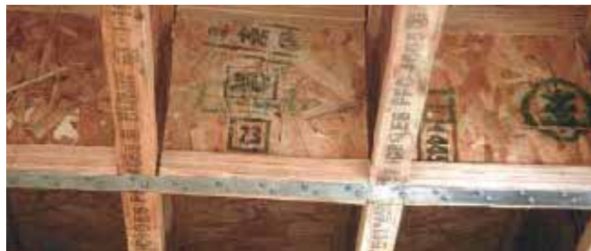
Figure 6. This collector was assembled from wood I-joint blocks and strapping. Ideally, the ends of the I-joint block webs would bear solidly against web fillers in the floor joists.
