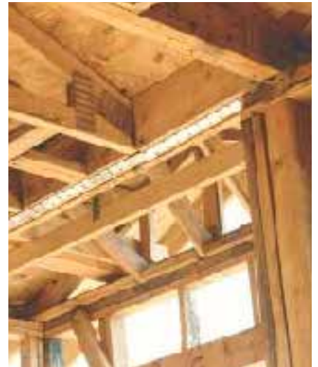
Figure 8. In this framing sequence, straps attached to the tops of shear walls are left hanging (top) until the installation of a blocked girder truss (above left), which will act as the collector for a section of roof. Finally, the straps are nailed to the bottom of the girder truss (above).
