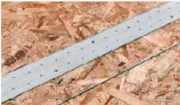
Figure 5. This strap was nailed to blocking below through the floor sheathing.
