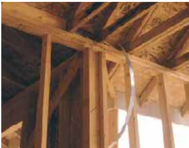
Figure 7. This strap, which runs from the top of a shear wall, will connect to the bottom of a roof truss above. Note that none of the trusses on the regular layout fell in line with the shear wall, so the builder had to add an extra off-layout truss to catch the strap. The roof sheathing will also have to be solidly nailed to this truss so that it picks up lateral forces in the roof diaphragm.
