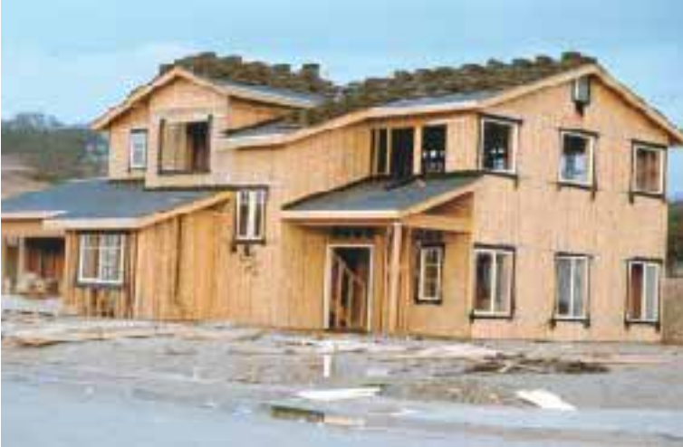
Figure 13. These photos were taken of two nearly identical houses in the same tract and illustrate how a change in the engineered plans can render a collector useless. In House A, which was built according to the stamped plans, the section of roof in the small front-facing gable is tied by a strap running from a shear wall at the corner of the house to a collector truss running in the same direction (see plan).
