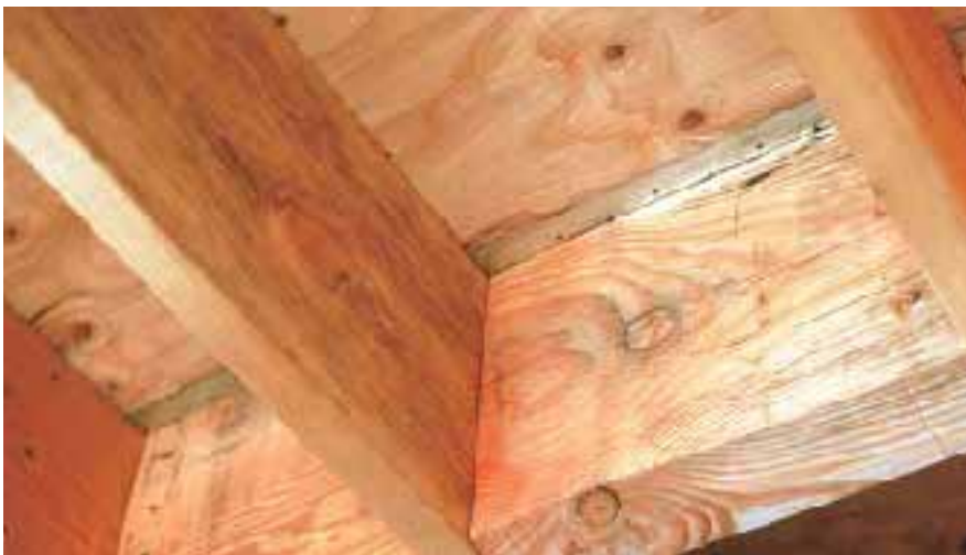
Figure 4. This strap was installed from the top before the floor sheathing was nailed down. The carpenter routed out the tops of the framing members to avoid a bulge in the carpeted floor above.
