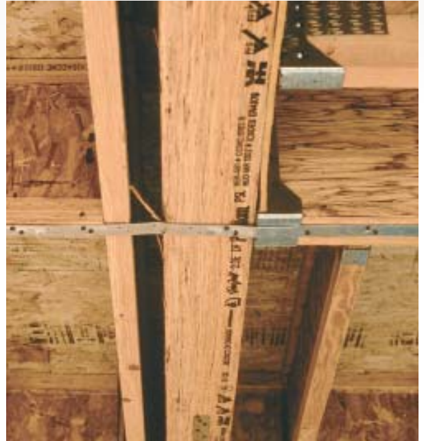
Figure 11. The missing block in this collector between the girder and the I-joist to its left could prove costly in an earthquake: The back-and-forth cycling of the quake will smash the two members together, folding and stretching the strap below until it fails.
