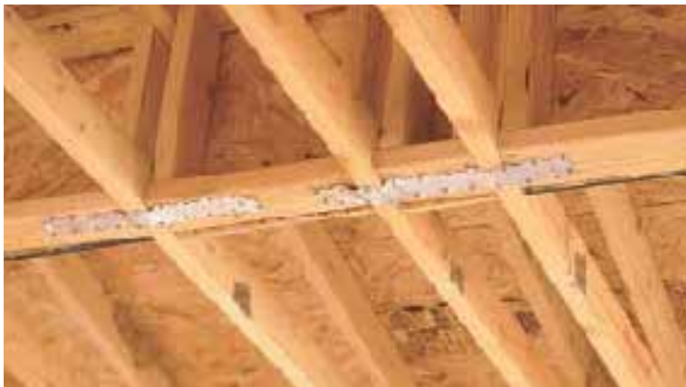
Figure 9. These photos illustrate a common mistake in building collectors — using many short straps instead of one long one. Each short strap must carry the cumulative load to that point in the collector, meaning that the strap near the end of the collector is likely to fail.
