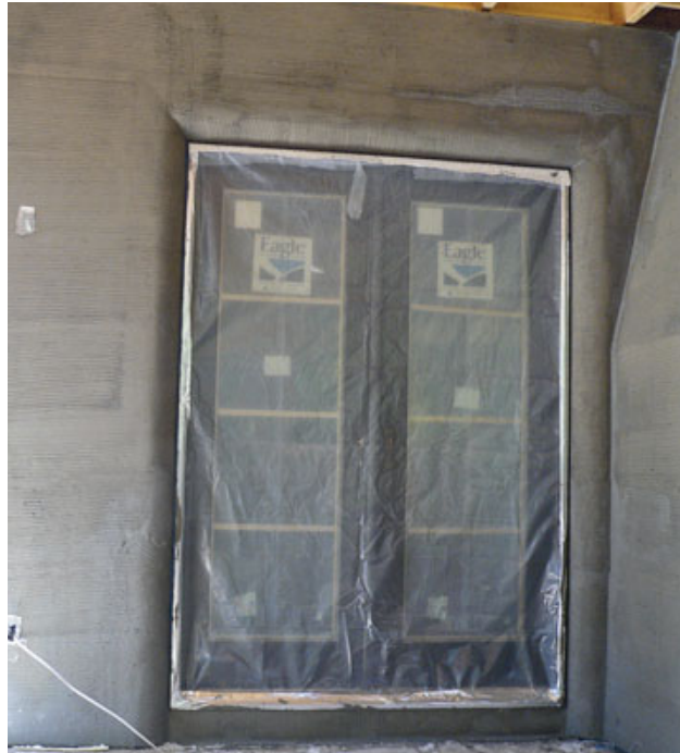
Figure 4. Base-coat application can begin after the foam has been leveled with a rasping board and abraded with a grit-welded float. Inside and outside corners get a double thickness of reinforcing mesh bedded in the base coat (far left). To help with adhesion, these walls received a second base coat, which was then scratched with diamond mesh lath (left).
