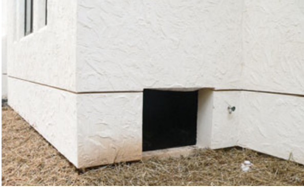
Figure 6. Expansion joints are needed in EIFS cladding wherever two dissimilar substrates meet, such as at the foundation.
