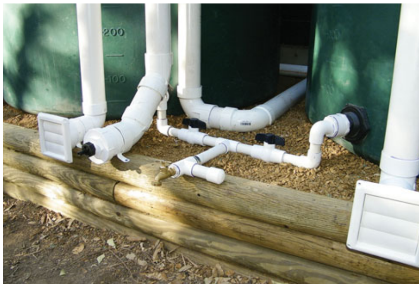
Figure 6. The overflow pipes on this nonpotable system terminate at louvered vents (designed for clothes driers), which open as the water escapes, then close to keep insects out. The black fitting to the right of the louver (above) is the dripper valve that drains the first-flush diverter. This simple system has no pump; water is drawn by gravity from the hose bib between the tanks.
