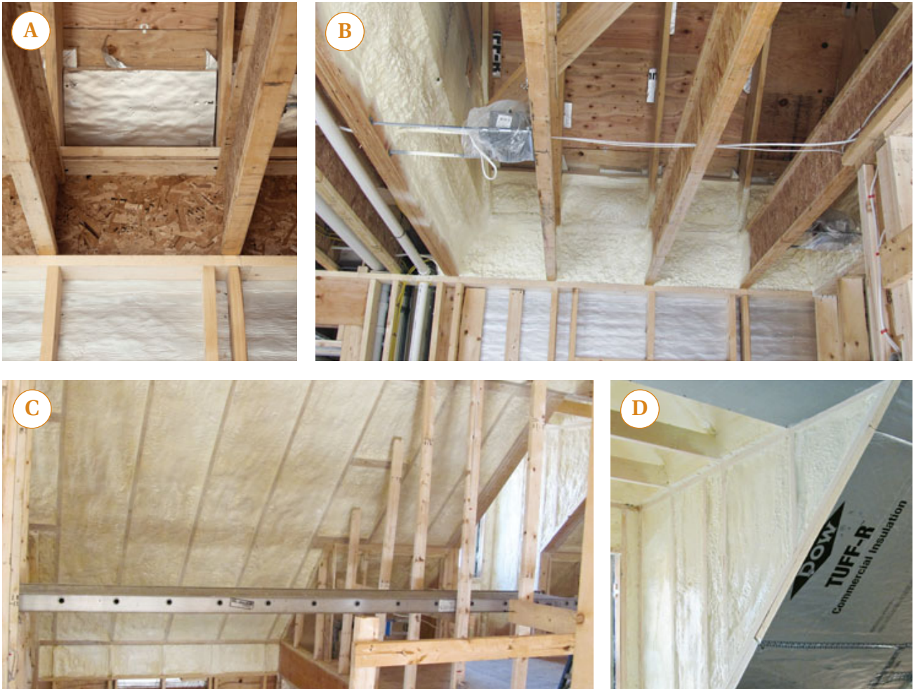
Figure 5. Foam-board vent baffles prevent wind-washing of the cellulose insulation in the attic ceiling areas (A). A 3-inch layer of spray foam effectively air-seals the vent baffles against the framing and insulates the rim joists to about R-18 (B). Sloped ceiling rafter bays were fully baffled with 2-inch foam board, then filled with closed-cell foam (C). Note the insulated rim joist and squash blocks below the single top plate. A layer of 2-inch R-13 foam board completes the sloped ceiling insulation, yielding a total approximate R-value of 70 (D).
