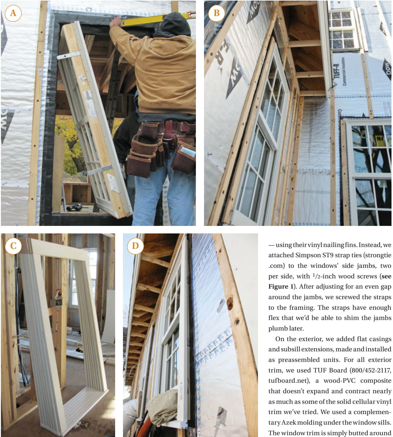
Figure 1. Metal strap ties screwed to the jambs secure the windows to the framing (A). Exterior window casings were fastened over the 1x3 siding vent strapping (B). The author preassembled the window trim using composite lumber and PVC subsills (C). Water that bypasses the siding and trim is shed by the foam sheathing's foil face (D).
