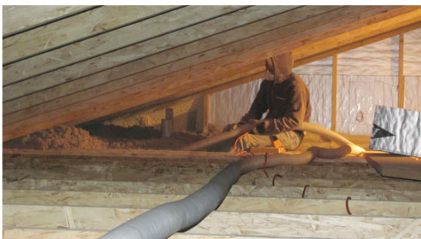
Figure 8. Dense-pack cellulose insulation was blown behind a permeable membrane stapled to the studs (top). Attic ceiling areas were sheetrocked first to support the insulation. Attics received a 16-inch layer of loose-fill cellulose with an R-value of 65 (above).
