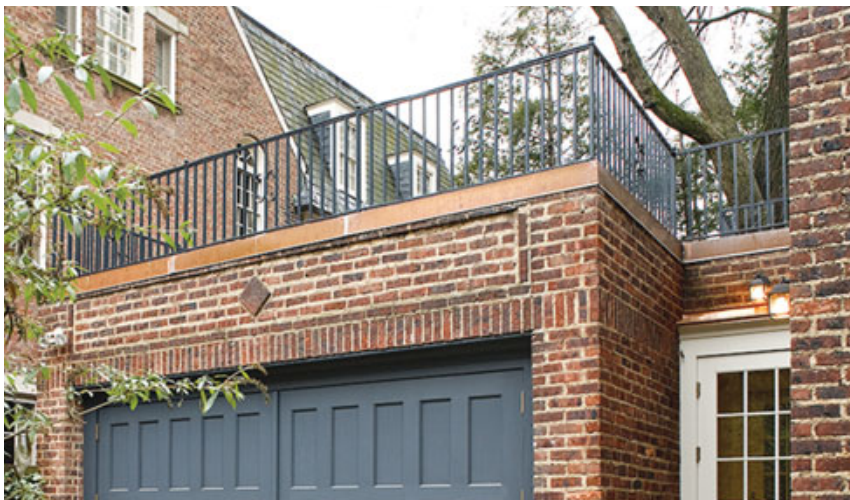
Figure 2. New copper flashing fitted around an iron deck railing serves as a waterproof cap over the parapet.
