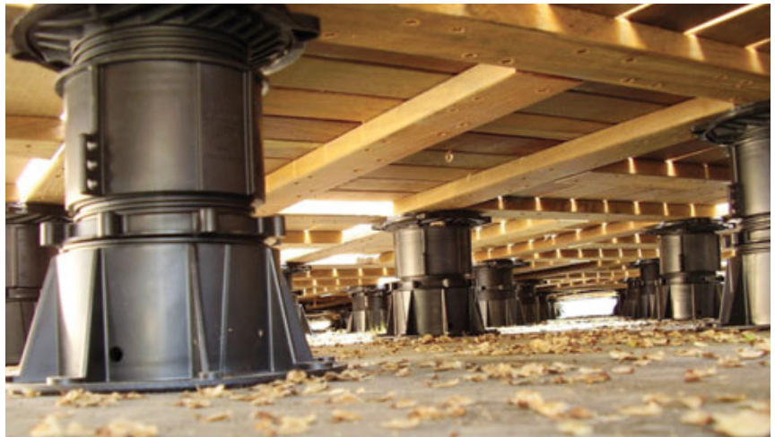
Figure 3. A series of adjustable plastic pedestals, each rated for a 1,500-pound load, hold up the deck. This support system makes it possible to clean leaves and debris from under the deck, or make adjustments.
