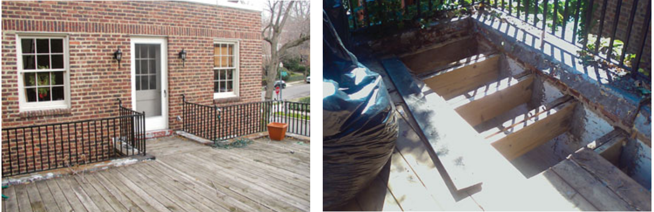
Figure 1. The existing pressure-treated deck (left) covered a leaking roof membrane and rotted sheathing. To reinforce the existing roof framing, the author sistered new joists alongside the old, supporting them in expanded masonry pockets (right). The old decking was replaced and a new EPDM roofing membrane installed.
