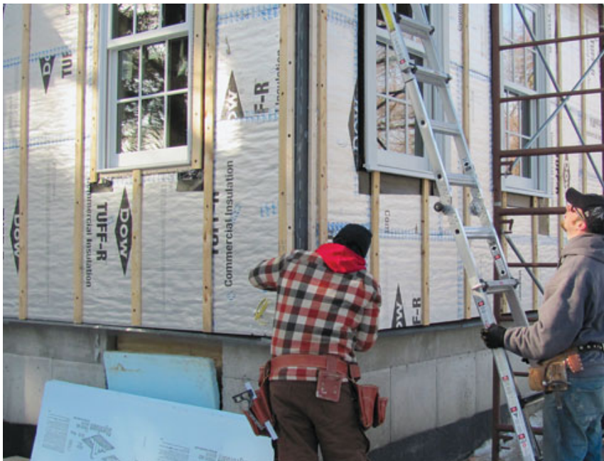
Figure 6. With the foam sheathing serving as a drainage plane, 1x3 vertical strapping creates a venting and drying space behind the siding. Additional strips around windows and doors provide separate backing for trim and siding.
