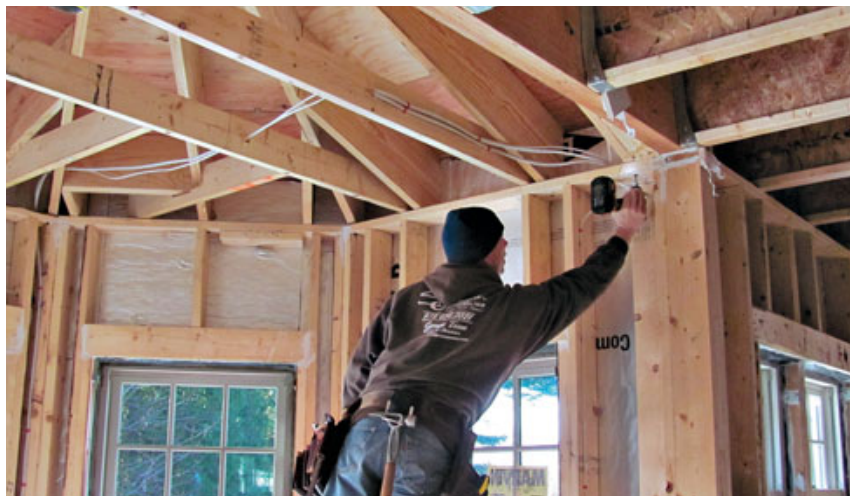
Figure 2. For the 24-foot lengths required to frame the main roof, the author used LSL (laminated strand lumber) rafters and collar ties in place of old-growth dimensional lumber (top). The floors are framed with 14-inch I-joists on 2-foot centers. TimberLok structural screws replace metal ties for faster, code-approved rafter hold-downs (above).
