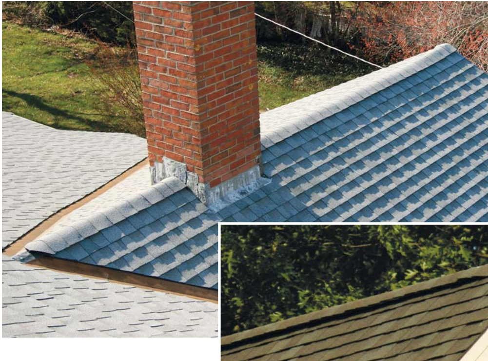
Figure 9. Vented ridges look best when the shingle-over material runs all the way to the ends (left). Proper end closures are created by folding a shingle over the ridge opening underneath the vent material. The common method of stopping the vent shy of the end creates a pinched look and draws attention to the ridge (below).
