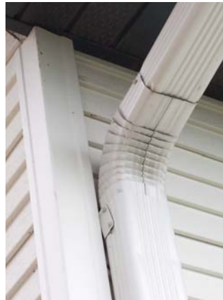
Figure 7. Concealing the seams on downspouts makes for a better-looking job, though it's not possible to do this with an elbow (far left). Installing the mounting clip at the joint between the elbow and downspout does double duty: It secures the downspout to the building and locks the joint together (left).
