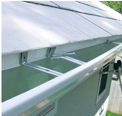
Figure 5. Slipping the back of the gutter beneath a properly installed drip-edge (far left) prevents rainwater from running behind the gutter (left). When the gutter slopes beneath the drip — or there isn't one — an apron flashing serves the same purpose (below).
