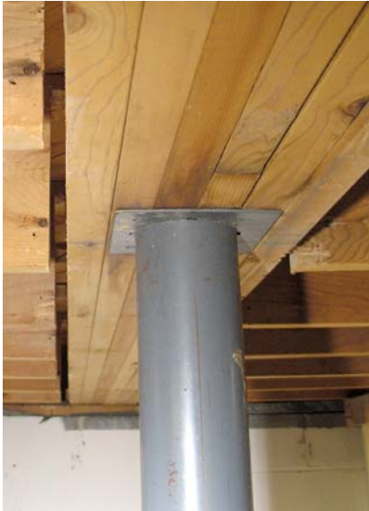
Figure 2. After temporarily supporting the floor, the crew cut the joist ends away from the girder, creating a channel for the two T-shaped steel beams to slip into.
