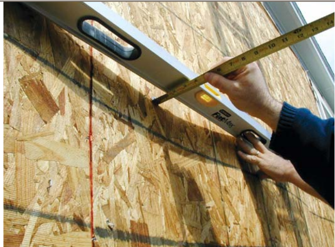
Bowed framing and wall sheathing installed without \frac{1}{8} -inch expansion gaps between the edges and ends of every panel can lead to panel buckling and wavy walls.
