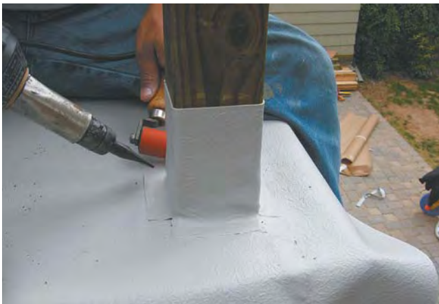
Figure 5. Watertight joints are made by heating overlapping edges of the membrane with hot air from a heat gun and then applying pressure to the seam with a hand roller (top). The collars around the posts are also heat-welded to the deck membrane (above).
