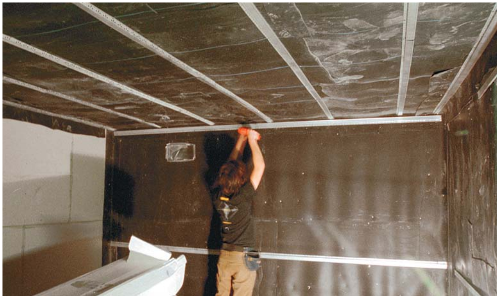
Figure 3. Mass-loaded vinyl fastened to the first layer of drywall deadens sound transmission through the walls and ceiling. On top, resilient channel is installed to receive the finish drywall layer.
